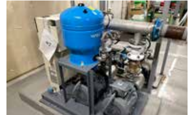
Factory water supply pump Kangawa Works
