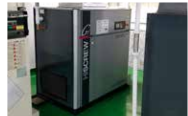
Compressors at the Fujiyama Works
